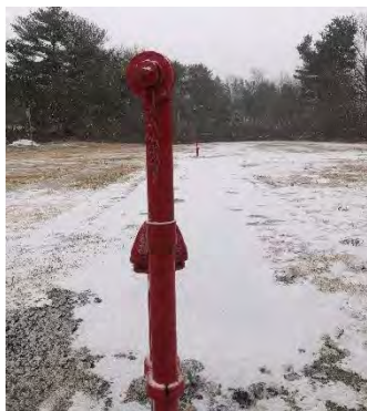
New spigots in the garden site at the Route 33 city-owned NH Ride Share parking lot (photo taken in early March)
